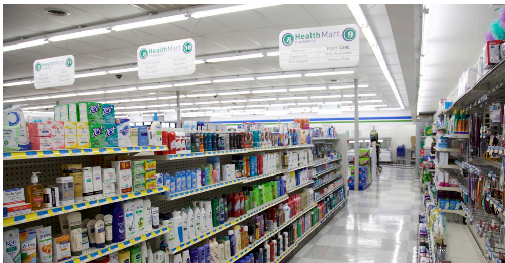
The LED lighting upgrade at Shrivvers Pharmacy's Nelsonville location
