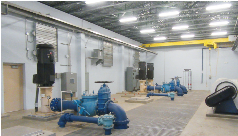
Occupancy sensors and high-efficiency lighting helped cut Del-Co's energy usage in half
